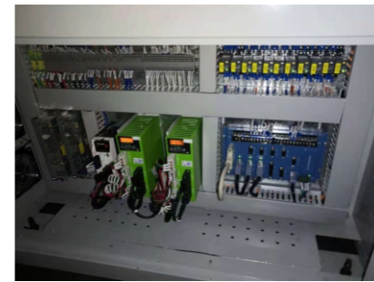
The electrical wiring is neat and consistent
