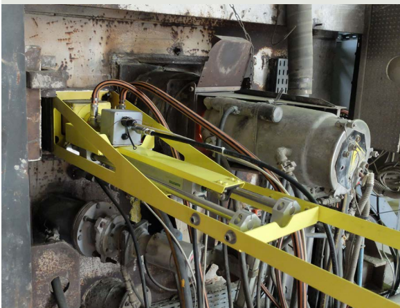
→ Pyroscan installed close to the kiln burner
