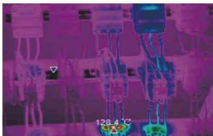
Distribution cabinet detection
